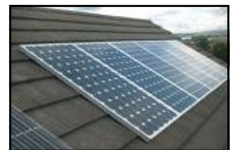
Solar Photovoltaic Panels
